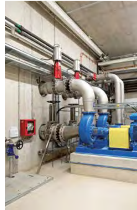
The pumps in the cellar move the water from the backflow basin to tanks located in the building's attic.
